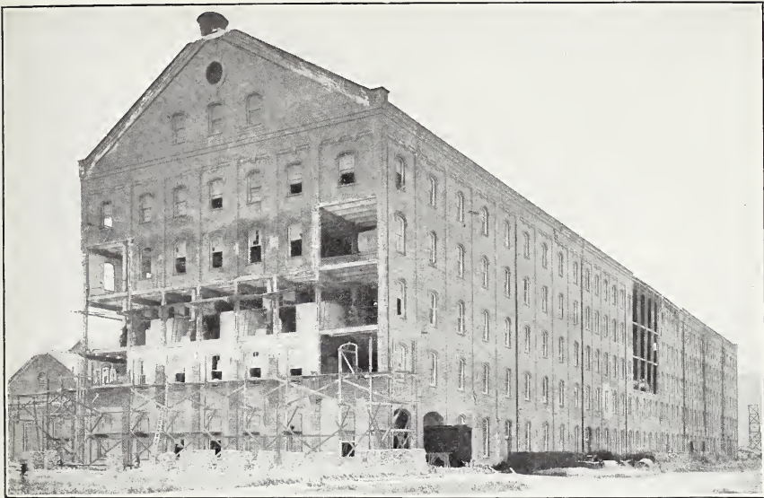
A. EFFECT OF EARTHQUAKE ON THE END AND THE INSUFFICIENTLY BRACED CENTRAL PORTION OF A BRICK BUILDING, SPRECKELS'S SUGAR MILL, ABOUT 4 MILES SOUTH OF SALINAS.
